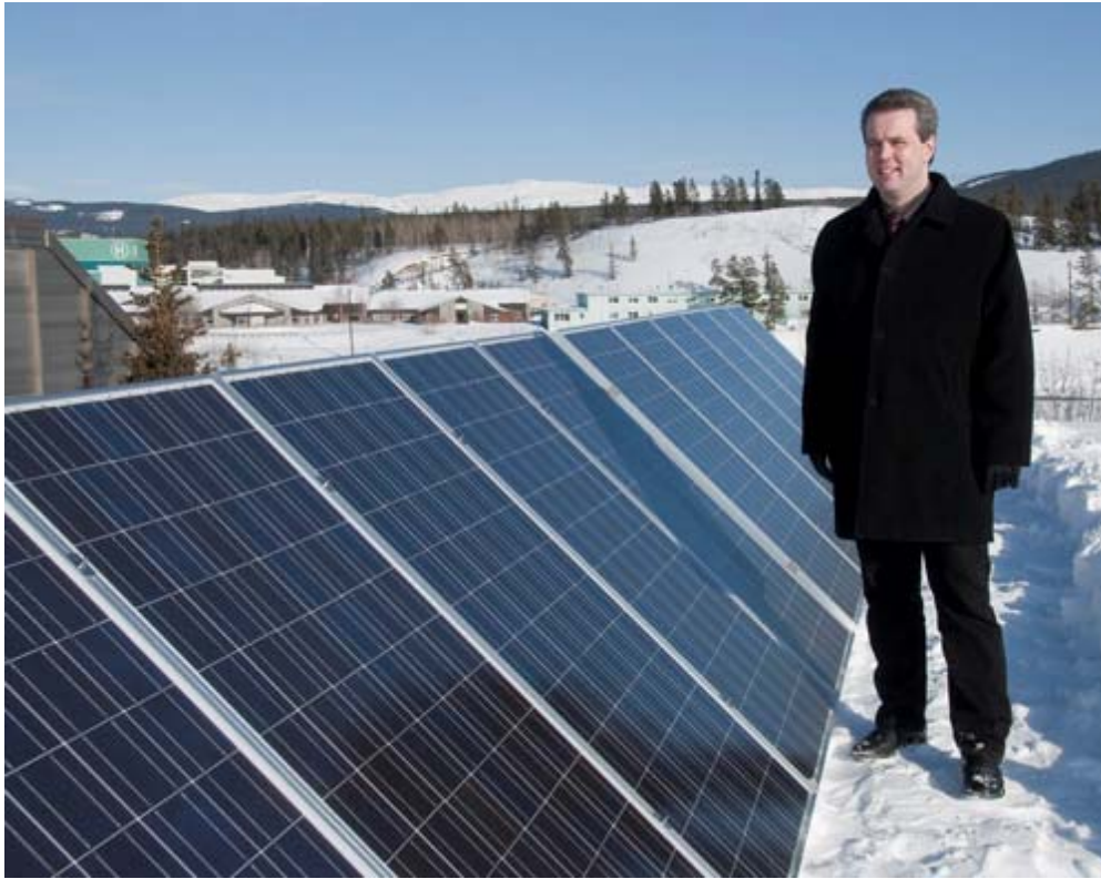
Energy, Mines and Resources Minister Brad Cathers with the photovoltaic solar panels atop the Yukon Government Administration Building
